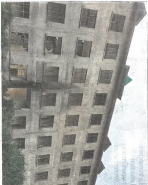
The Government Degree College building remains incomplete.
