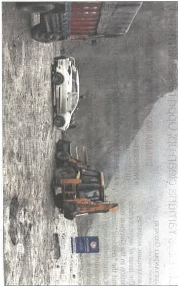
Flashfloods occurred at Pagal Nullah on the Manali-Rohatang road. VIDEO GRAB
