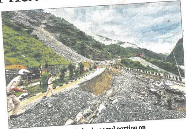
Security personnel check the damaged portion on Chandigarh-Manali highway in Mandi district of Himachal Pradesh after a landslide in July.
